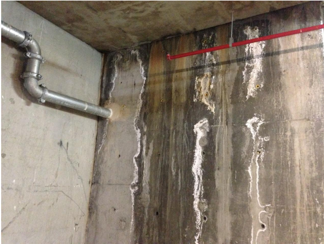
Figure 3: Basement Wall Water Ingress in Liverpool NSW
