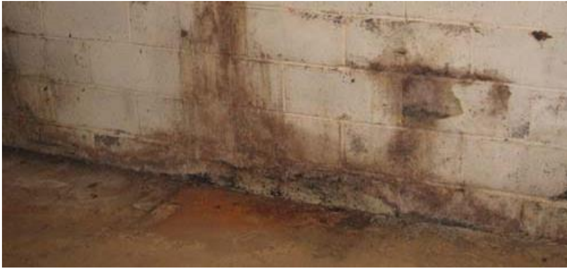
Figure 4: Block Wall Water Ingress Causing Decay
